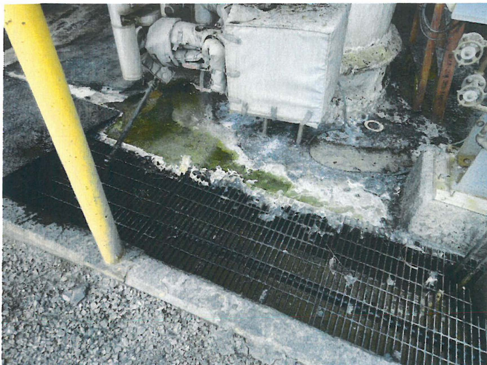
Photo #13: Liquid material escaping from a valved pipe end and into the sump, at the C5 Unit.
