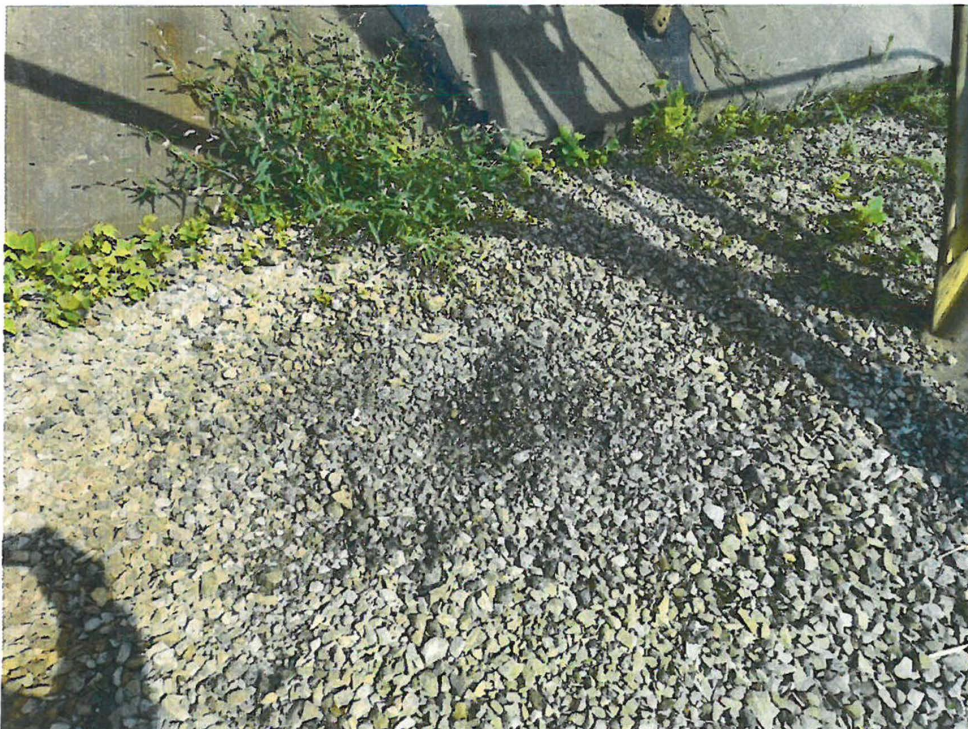
Photo #25: Stones covered in material that leaked from overhead piping, outside the 160 Battery containment, specifically, behind tank 161. Same location as Photo #1. Photo #25 taken on the morning of 08/15/2018 (Day 2 of inspection).
