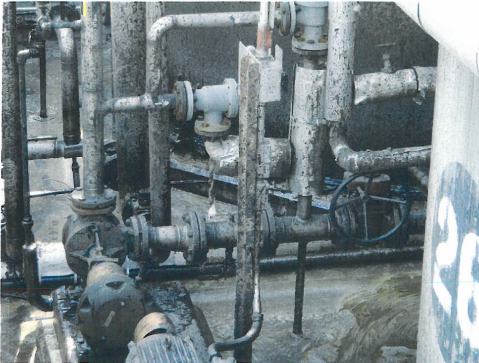
Photo #18: Closer view of the semi-liquid material from Photo #17, at the base of Tank 27
