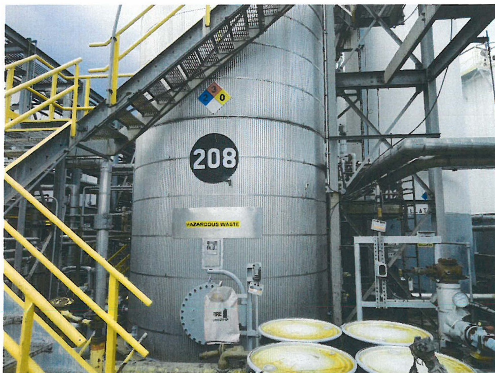
Photo #22: Closer view of Tank 208 labeling
