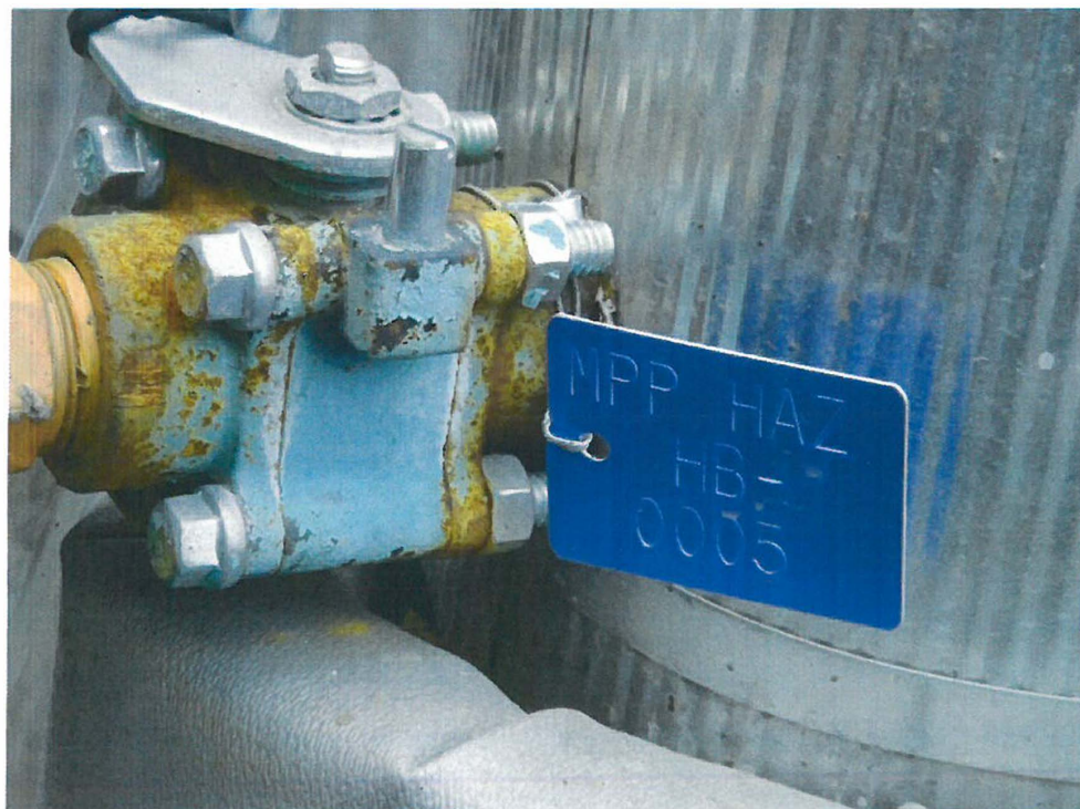
Photo #23: Metal tag "MPP Haz HB-0005" on valve attached to Tank 208. Equipment identification, as part of the Facility's LDAR program.
