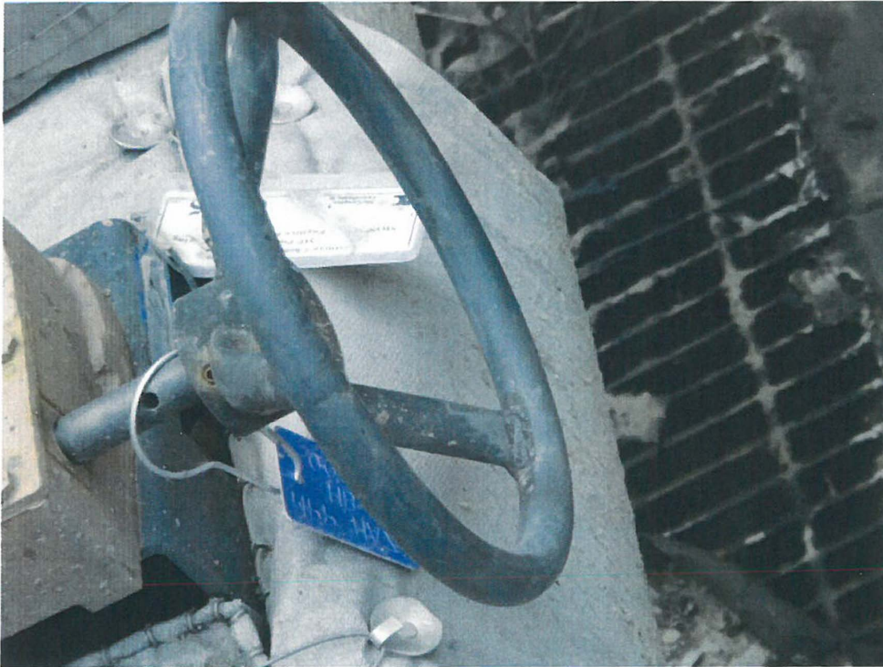
Photo #24: Metal tag “MPP Haz HB-0006” on valve associated with Tank 208. Equipment identification, as part of the Facility’s LDAR program.
