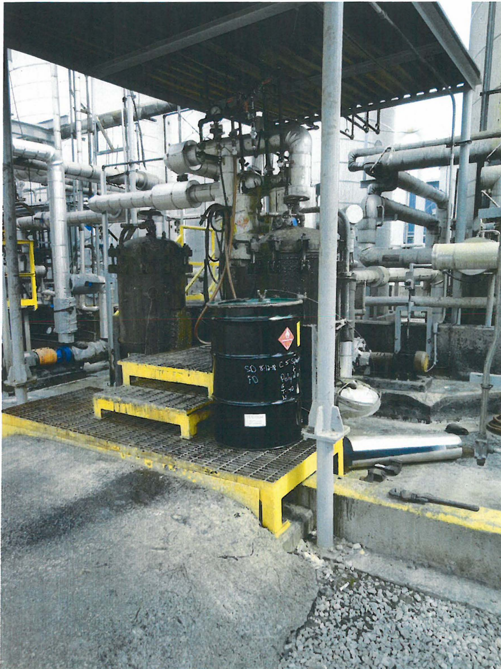
Photo #26: (1) closed 55-gallon container labeled as hazardous waste "C5 Spent Filters and Poly'd (sic) Oil", and start date 8/12/18, at the 500 Battery containment.
