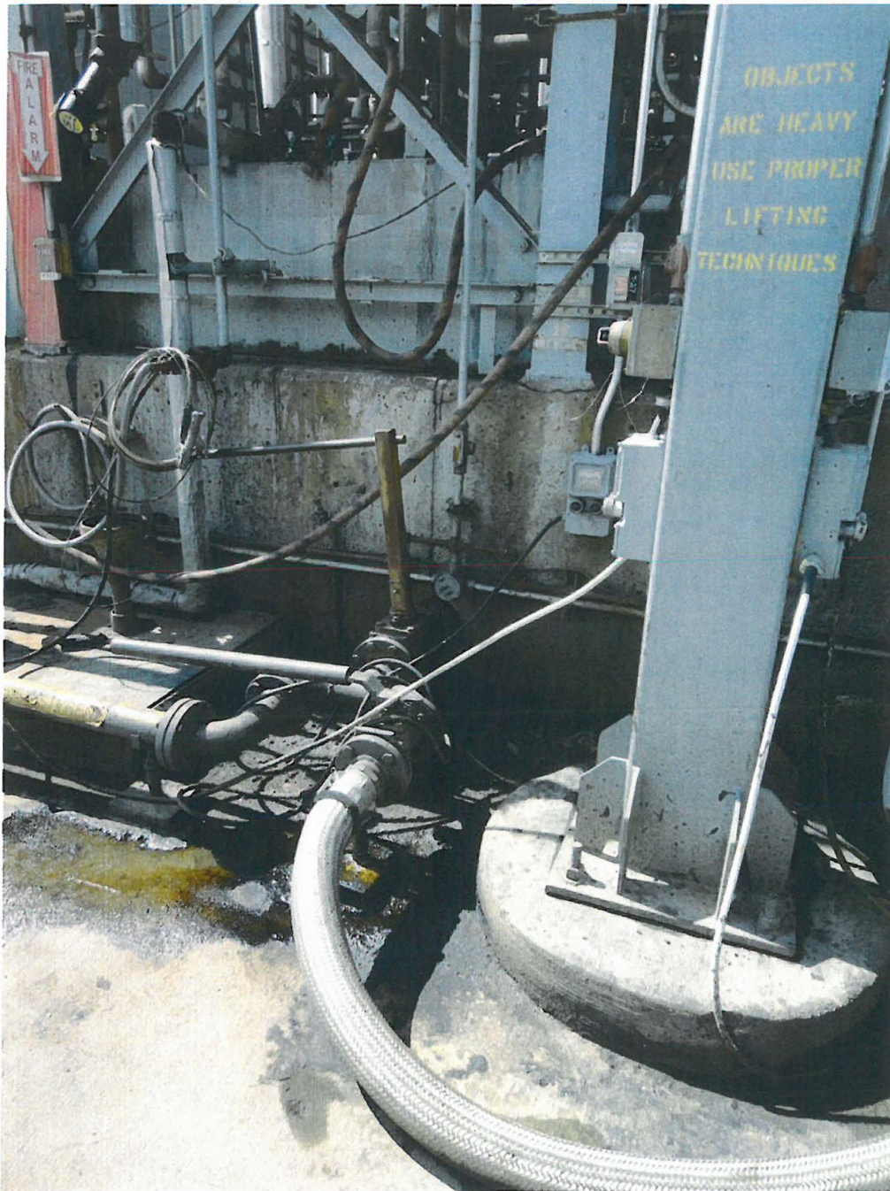
Photo #15: Lower Water White Truck Pad, external east side of Battery 20 Dike, liquid actively leaking from a stainless steel braided hose connected to a pipe.
