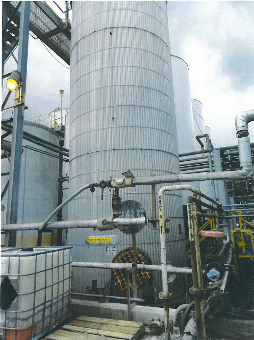
Photo #20: Tank 265, labeled with "Out of Service".
