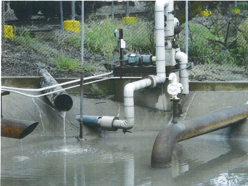
Photo #7: Close-up of pipe discharging into pond from Photo #5.
