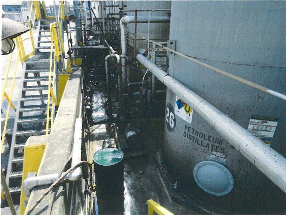
Photo #17: Base of Tank 26 (foreground, right) and Tank 27 (background, right) and floor of Battery 20 Dike with approximately 1/8" to 1/4" thick, sticky, semi-liquid material throughout.
