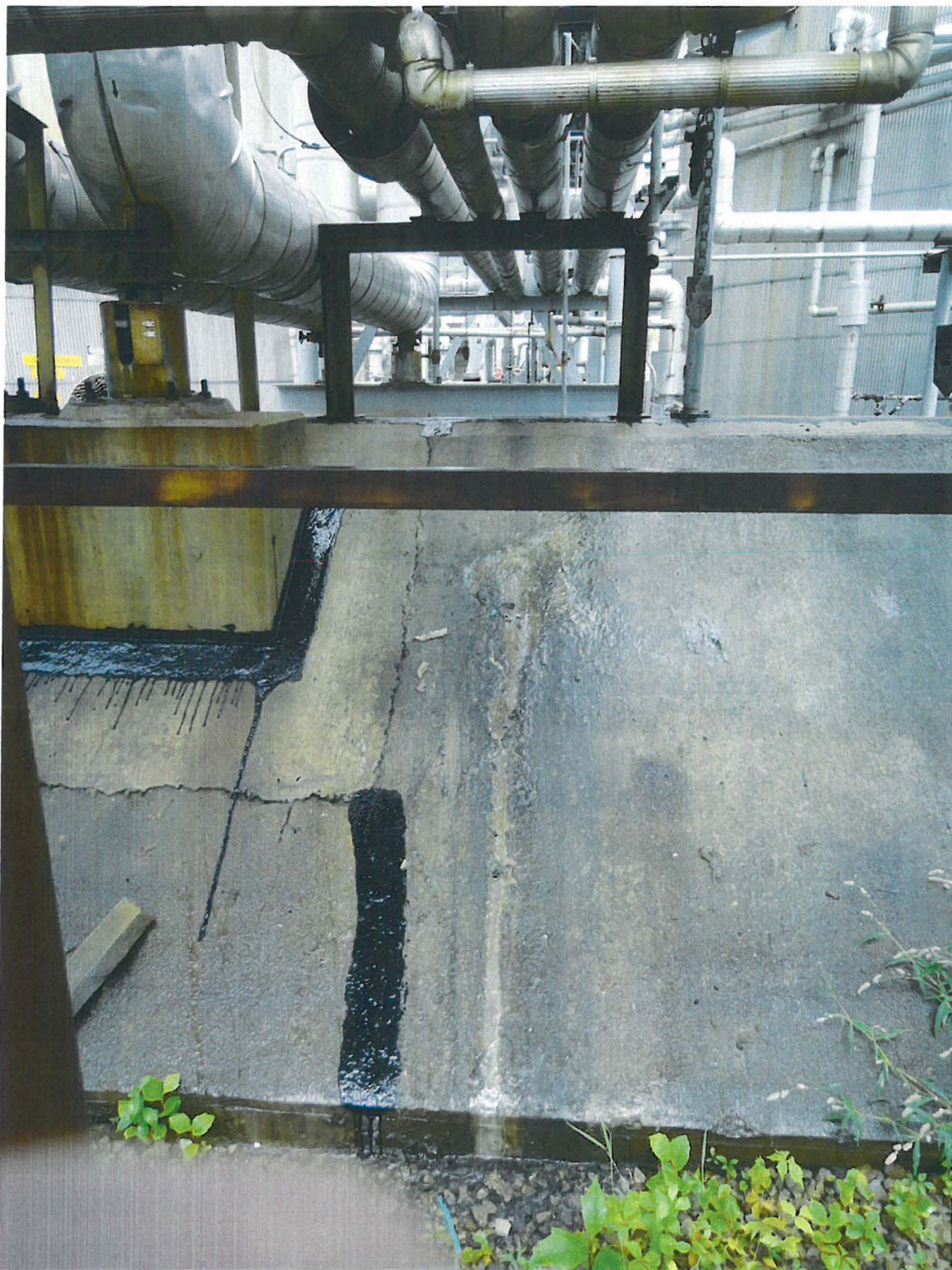
Photo #2: Spilled material on external berm wall of the 160 Battery containment.
