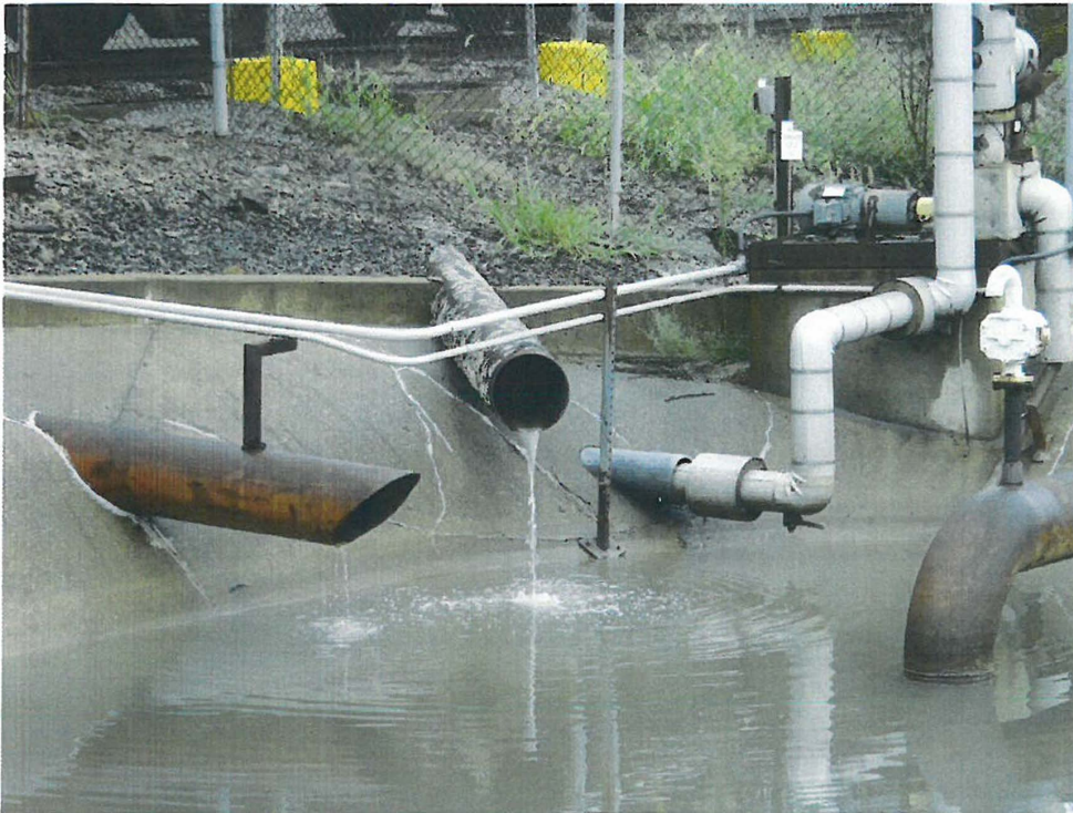
Photo #6: Close-up of pipe discharging into pond from Photo #5.
