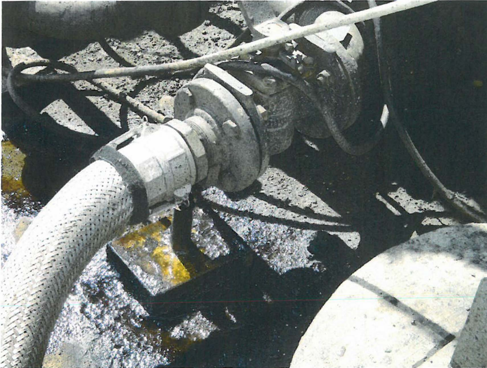
Photo #16: Close-up of actively leaking liquid from Photo #15.
