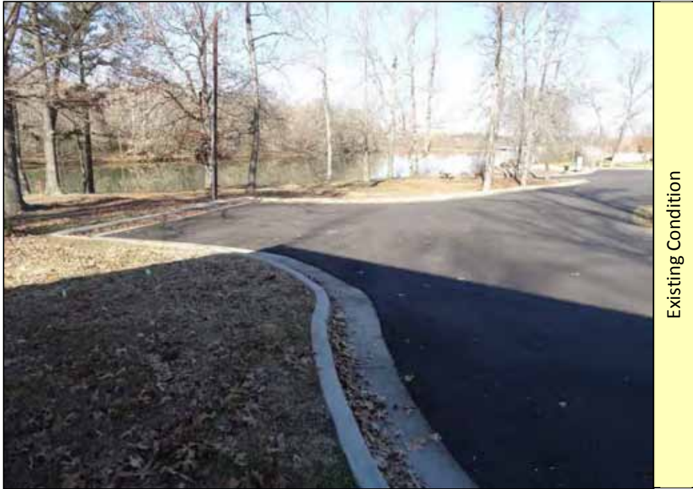
Picture 21: Existing parking spaces. Portion of curb to be removed to create accessible parking for future sidewalk to connect to the restroom and fishing platform.
