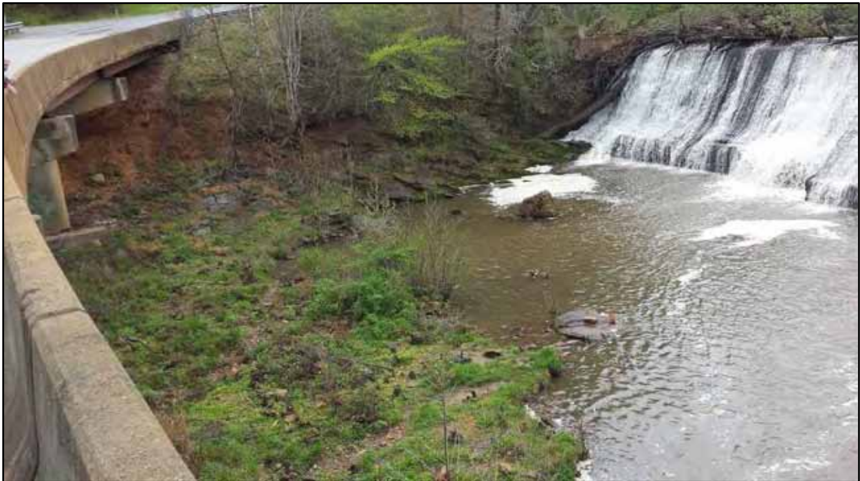
6. Over-widened channel and scour hole on right bank below Power Dam, view east (4/16/15)
