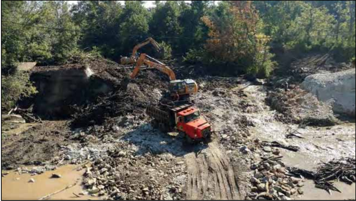
17. Breach nearly complete, woody debris removal continues, view southeast (9/8/16)
