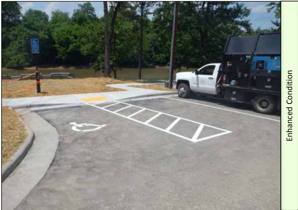
Picture 22: New accessible parking spaces with accessible sidewalk connecting to the restroom and fishing platform.
