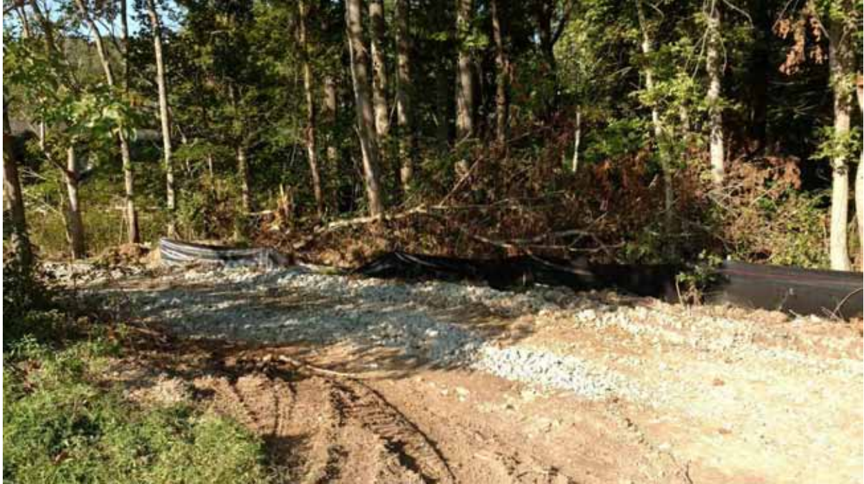
9. Access road down to floodplain causeway with silt fencing in place, view north (9/7/16)
