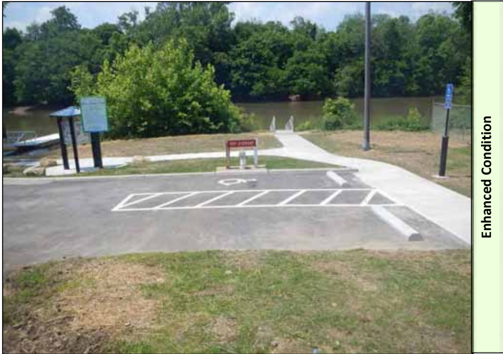
Picture 2: Added accessible parking and accessible sidewalk leading to the floating dock and canoe launch. Accessible sidewalk also leads to kiosk and courtesy dock.
