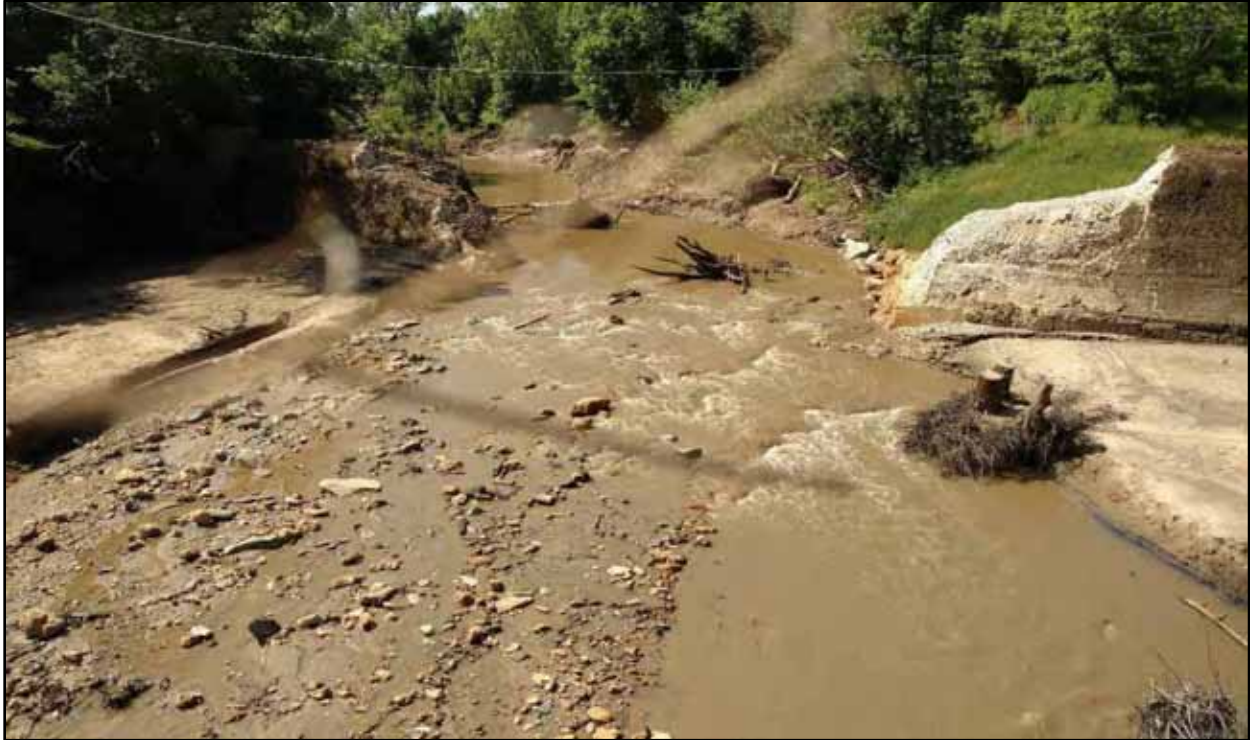
29. Cobble and gravel sediment transport through breach in dam (5/25/17)
