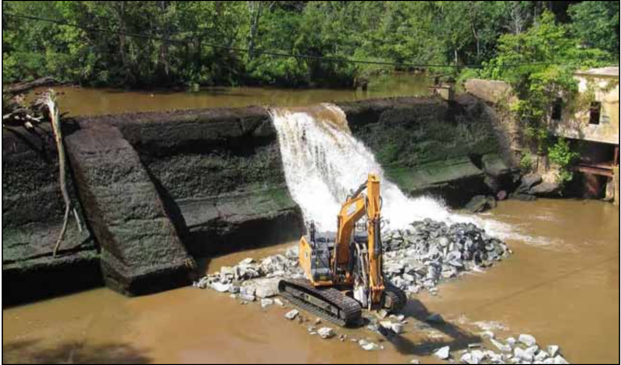
11. Initial dam breach, view southeast (8/29/216) (credit Franklin News Post)
