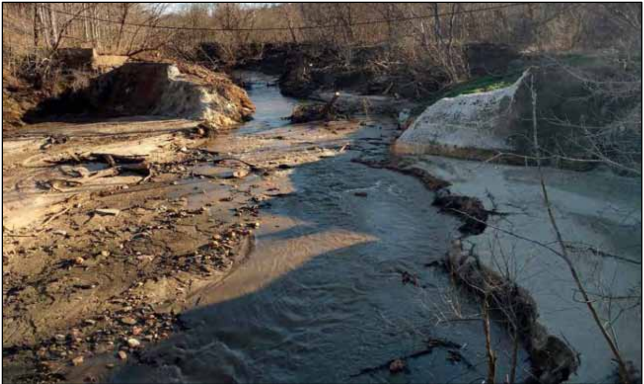
26. Floodplain deposition on left and right banks below breach (2/2/17)
