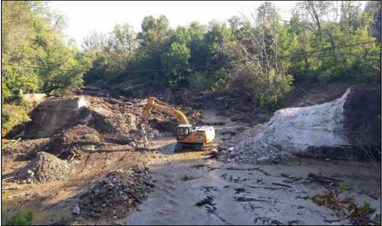
19. Fine-tuning breach opening and stockpiling of material in former scour hole to restore floodplain bench (9/12/16)
