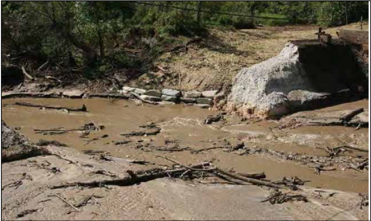
24. View of left bank upstream of dam after stacked stone toe, backfilling, and matting stabilization (10/5/16)
