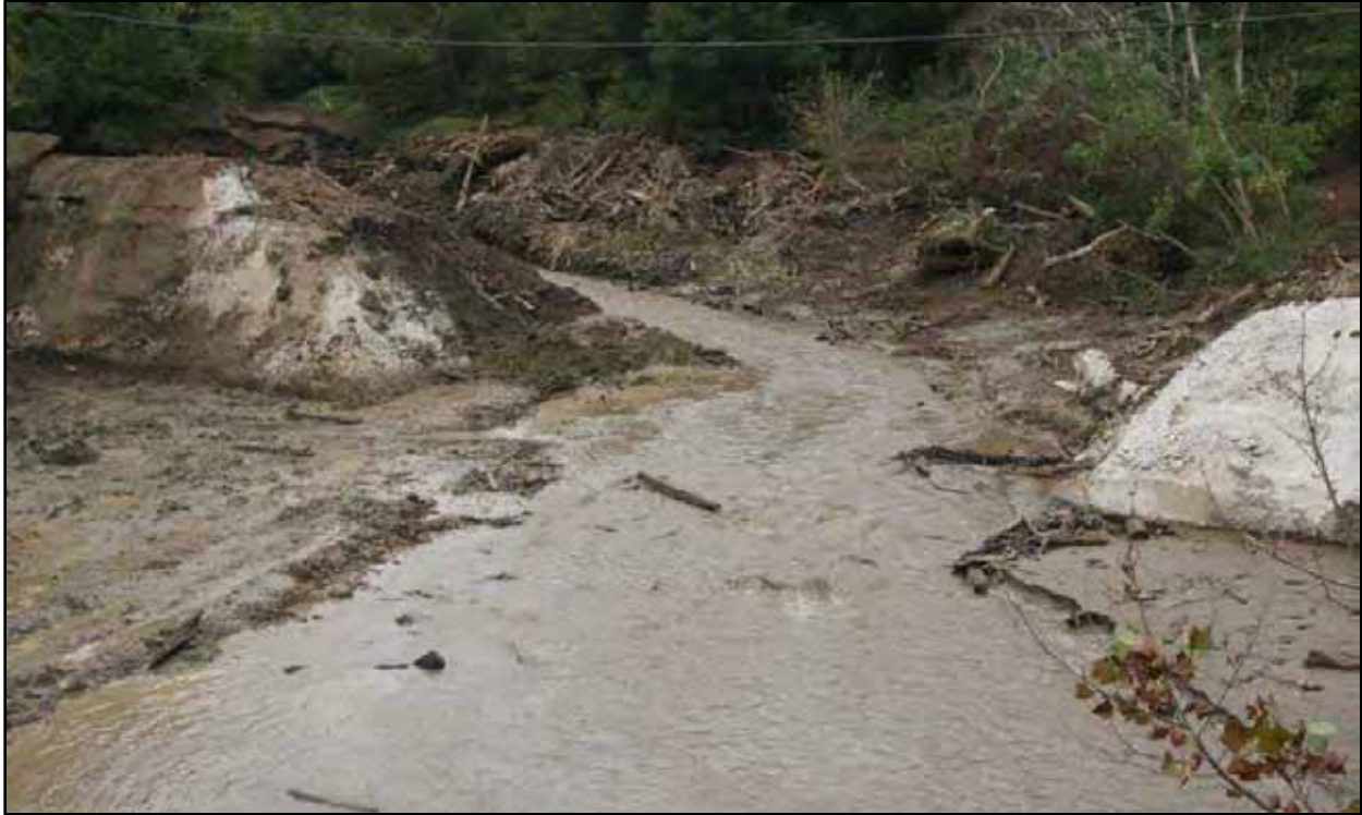
23. Sixty-five foot width base flow channel completed through Power Dam (9/22/16) (credit FORVA)
