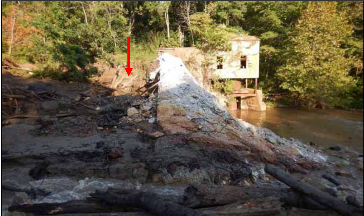
14. Exposure of existing scour hole (red arrow) above Power Dam, potentially leading to wetland headcut (9/7/16)
