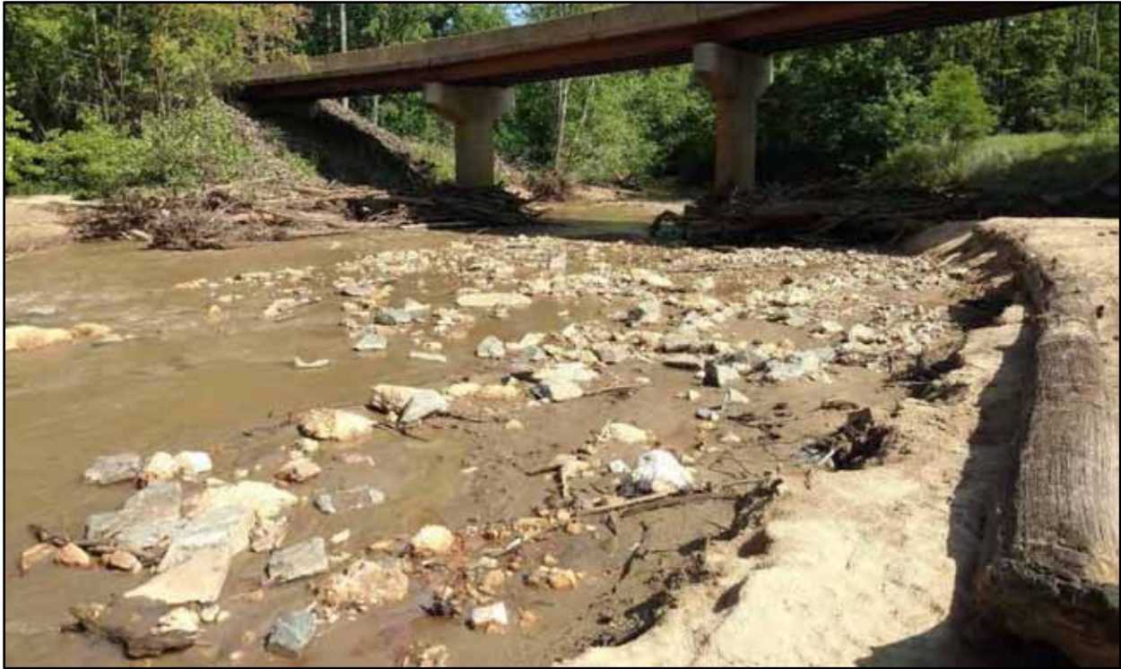
30. Additional coarse material deposition downstream between breach and Route 712 Bridge (5/25/17)
